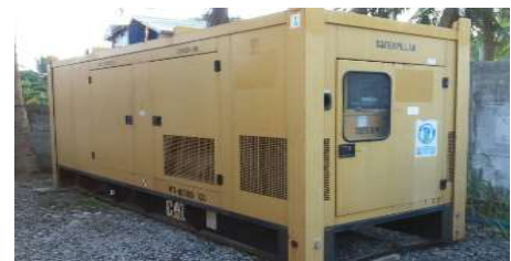
GENSET, CATERPILLAR, 230kVA
