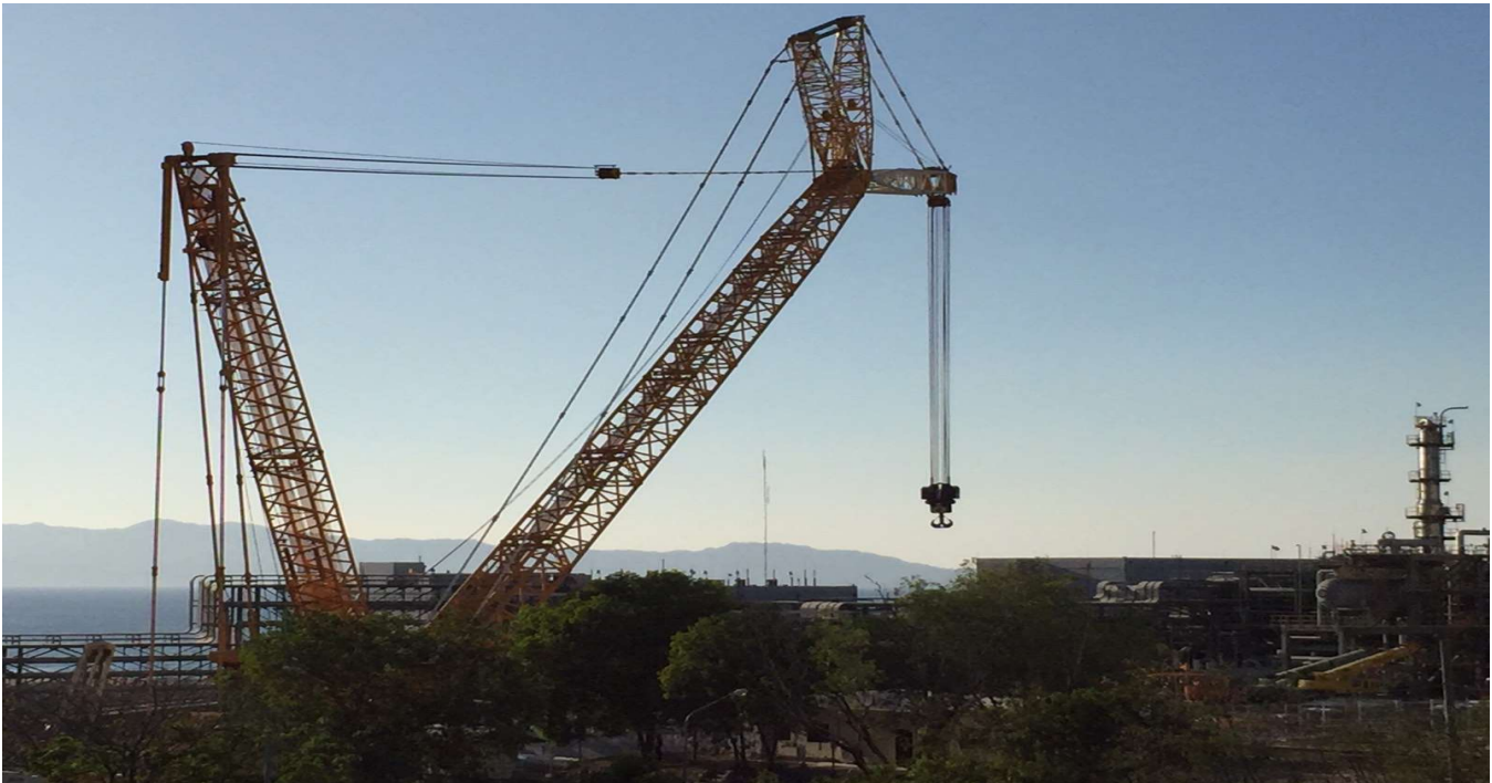
Complete Assembly of 1,350T Crane at the site, One of the biggest cranes brought in the Philippines
