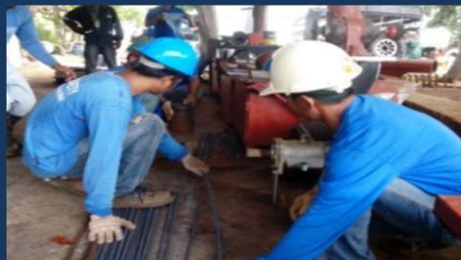
Fabrication of rebar's at fabrication shop for the construction of depot perimeter wall.
